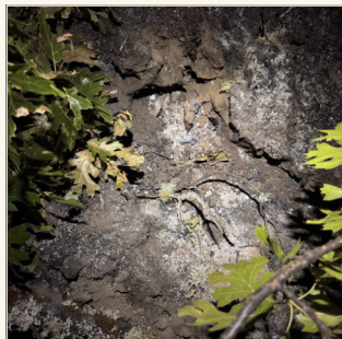
Stump hole hidden in timber, I-5, 4 Aug
